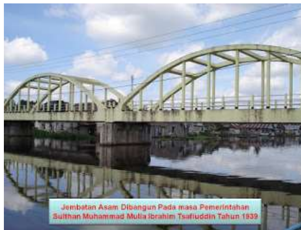
Figure 3. The Asam Bridge was built during the reign of Sultan Muhammad Mulia Ibrahim Syafiuddin in 1939
